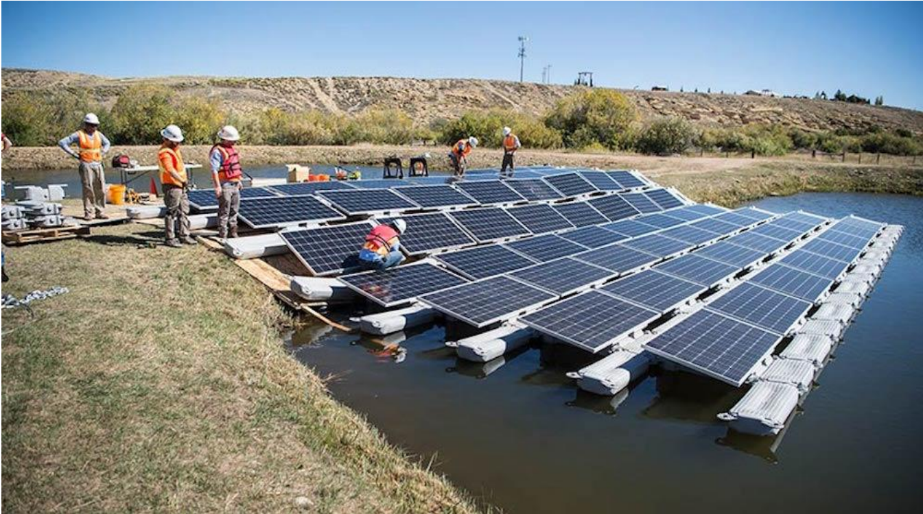
Figure 7 Example of floating solar technology being deployed.
