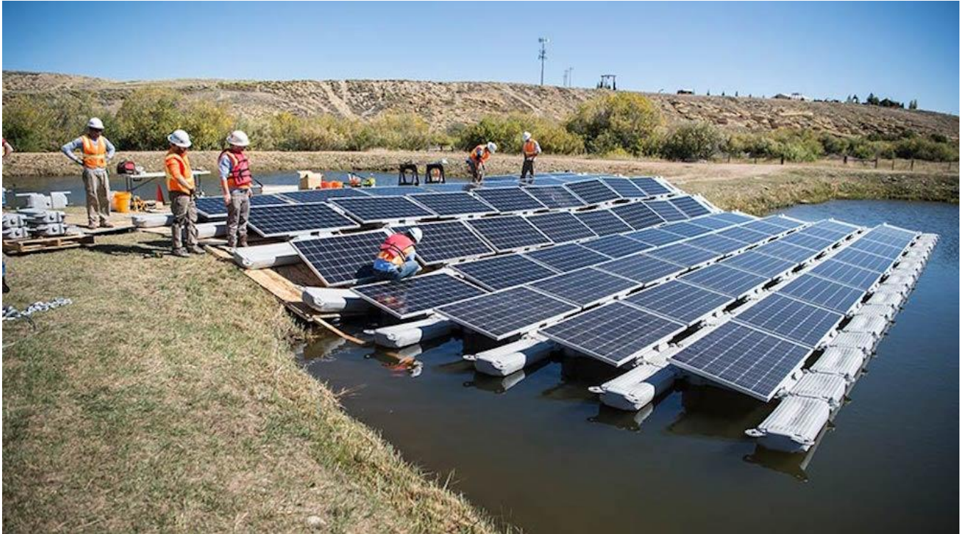
Figure 7 Example of floating solar technology being deployed.
